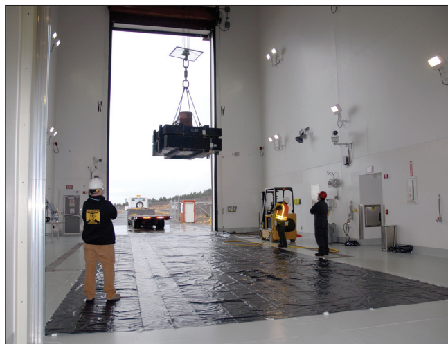
Proof testing of the crane in the Payload Processing Facility.
